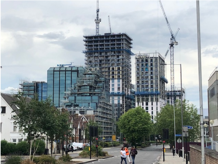
5. 3 of the 4 new buildings on the former Taberner House site have been topped out, whilst the 35 storey tower has reach 2/3rd of its final height
