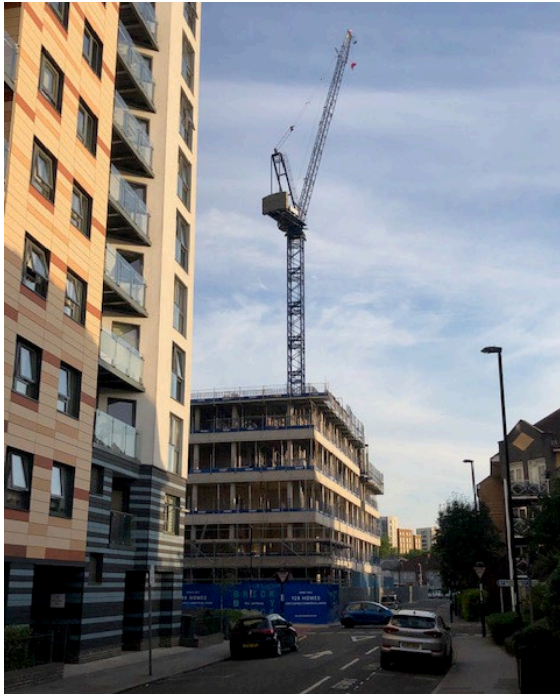
1. Brick by Brick's Kindred House tower on the former Wandle Road Car Park is rising rapidly
